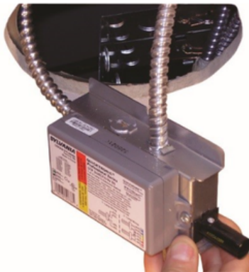
Fig. 39 Inner junction box cover (3D Cover #1242-18B) with mounted driver, removed for servicing below ceiling
